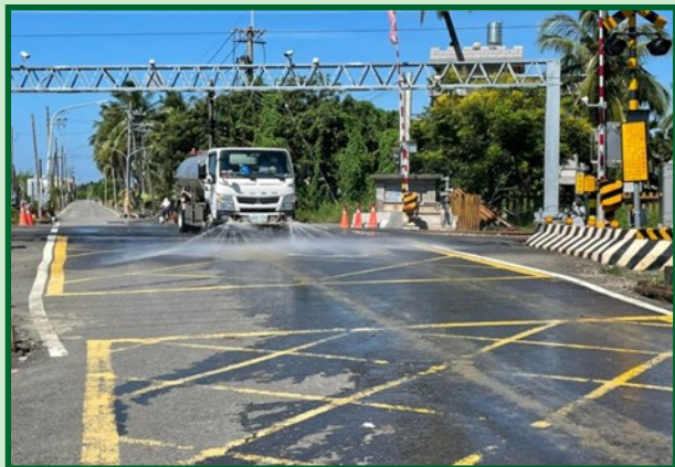
Washing and spraying water on the vehicle path in the work area
