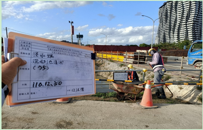
Desilting in the sedimentation tank
