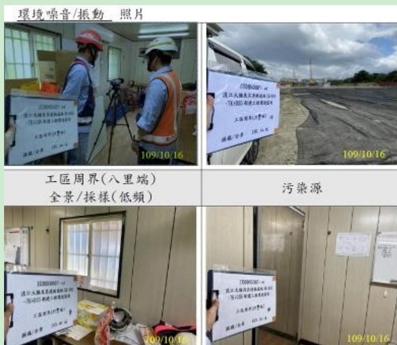
Noise and vibration monitoring panoramic sampling
