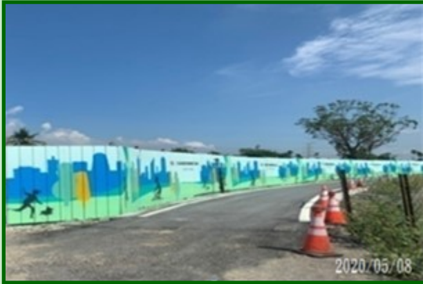
Set up anti-overflow seats on the perimeter of the work area to suppress the overflow of sewage
